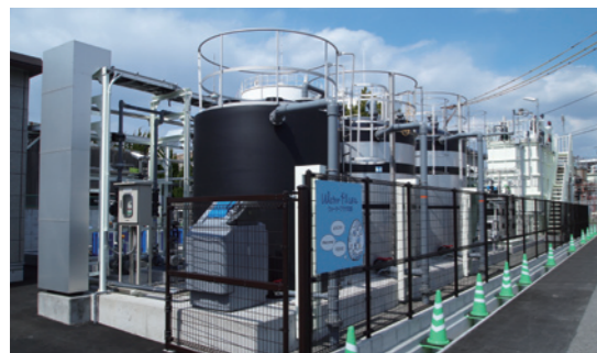
Start of operation: May 2011 Plant area: Approx. 640 m 2 Capacity: 400 m 3 / day Application of product water: Industrial water
