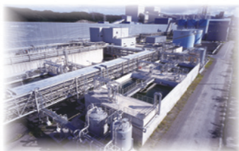
Industrial Wastewater Treatment Systems
