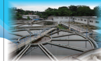
Water Purification Plant
