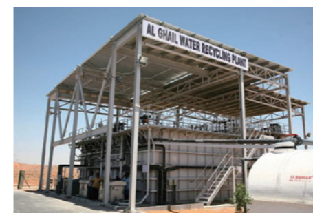
Start of operation: April 2010 Plant area: Approx. 3,600 m 2 Capacity: 2,000 m 3 / day Application of product water: Industrial, irrigation and landscaping water
