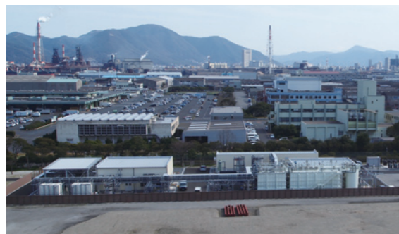
Start of operation: April 2011 Plant area: Approx. 3,600 m 2 Capacity: 1,400 m 3 / day Application of product water: Boiler feed water
