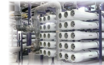
RO Membrane Facility
